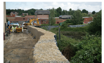
Construction crew fill Hesco units at Mythe water treatment plant in Tewkesbury
