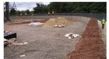
Hesco flood walls protect Walham electricity substation, Gloucester.
