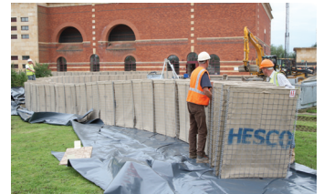
Construction crew extending Hesco units at Mythe water treatment plant in Tewkesbury
